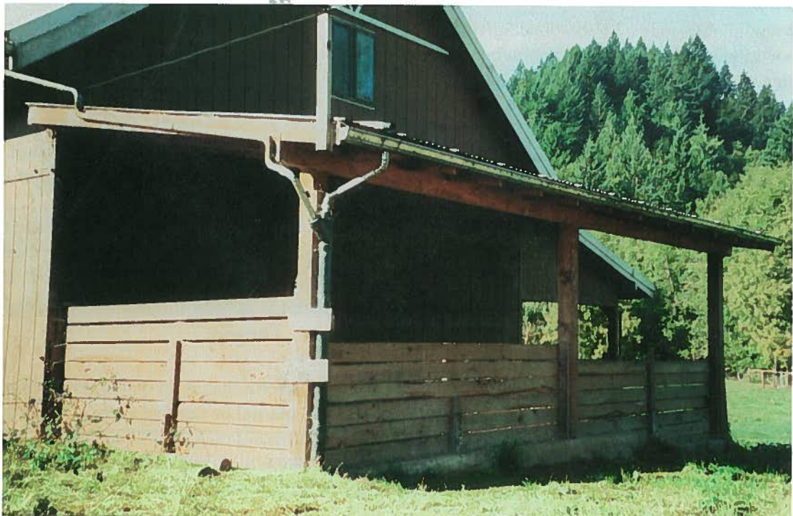
Lean-To Design Manure Storage Structure
